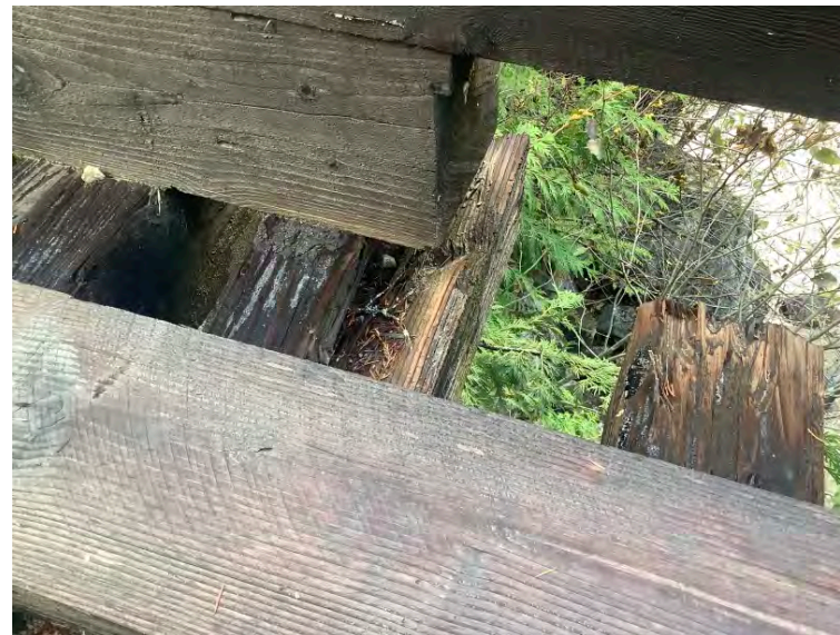
Damaged cross tie end
